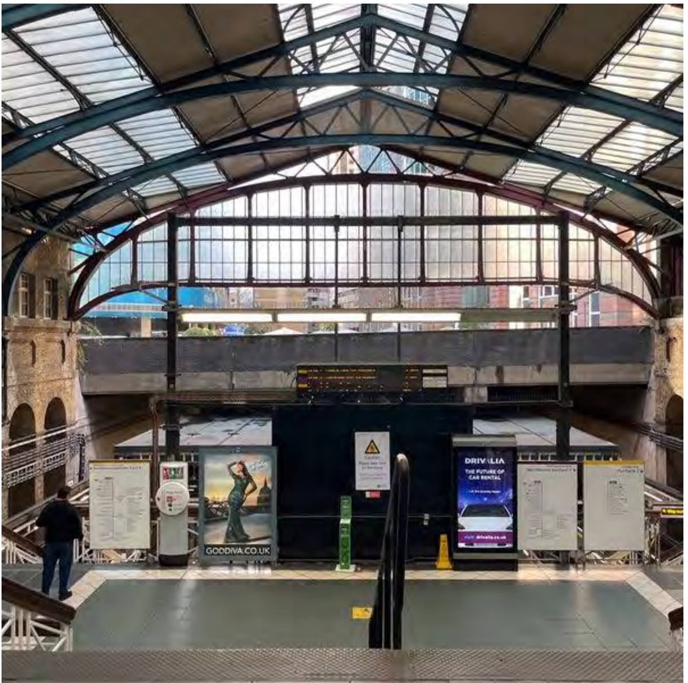
View looking north within the Victorian trainshed of Aldgate Underground Station, completed in 1876, with the cast iron span roof over the four platforms below (Credit: SAVE Britain's Heritage)
